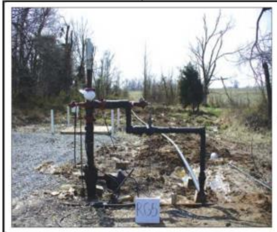
Figure 7 Surface wellhead and related piping of the injection well. Stainless steel lubricator at the top allows the cable connected to the downhole pressure and temperature sensors to enter the tubing.
