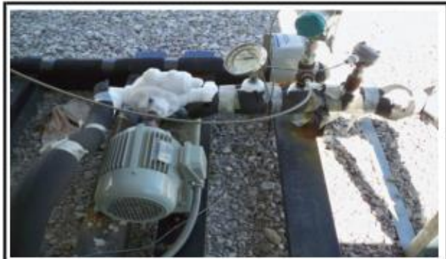
Figure 3 The booster pump (frosted over) site and the gray 1-hp motor (left foreground). A manual temperature gauge(circular dial) and Siemens pressure gauge (blue cap) to the right. The black hose connects to the storage tanks on the right and to the main pump on the left
