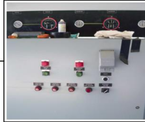
Figure 6 The pump control panel at site
