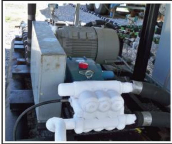
Figure 5 The CAT pump with input and output lines (frost-covered) in operation at site. The aluminium housing covers the belt and pulleys between the pump and crankcase (blue) and motor (grey).
