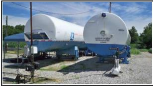
Figure 1 Two 60-ton (54-tonne) CO2 storage tanks at site. Data acquisition equipment in the left foreground
