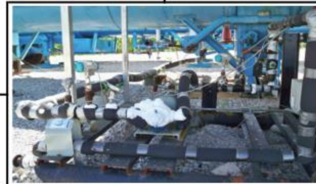
Figure 4 The booster pump skid at site. The pump (frosted over) is in the centre of the picture and the motor is the grey object behind it. The pipes are covered with black neoprene pipe insulation. The one on the left extends back to a storage tank.
